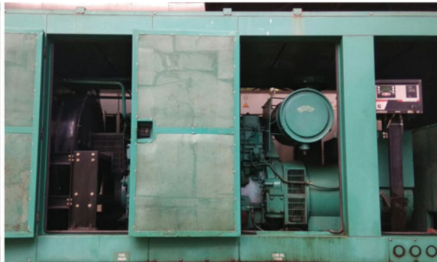
Diesel engine generator
