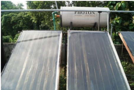
Solar water heater
